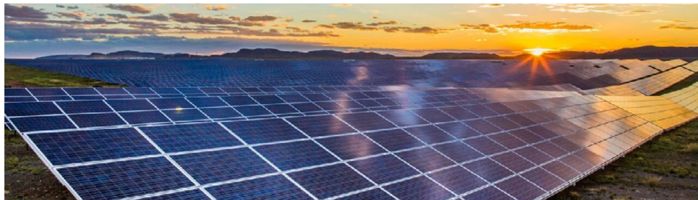
South African 50 MW PV Solar farm at De Aar-De Aar Solar Power
