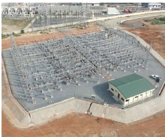
Collector Substation for Kpone Independent Power Plant- Ghana (2016)
